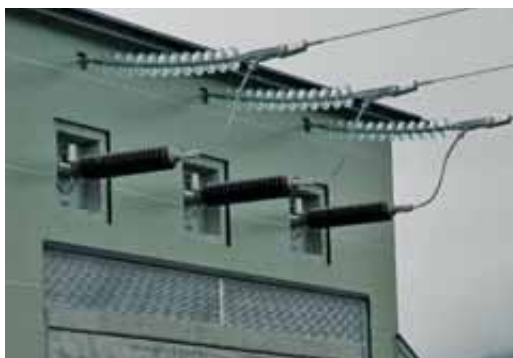
> Indoor/outdoor wall-bushing in a distribution substation.
