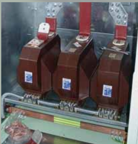
› ACM-12 Support type transformer for primary distribution switchgears.
